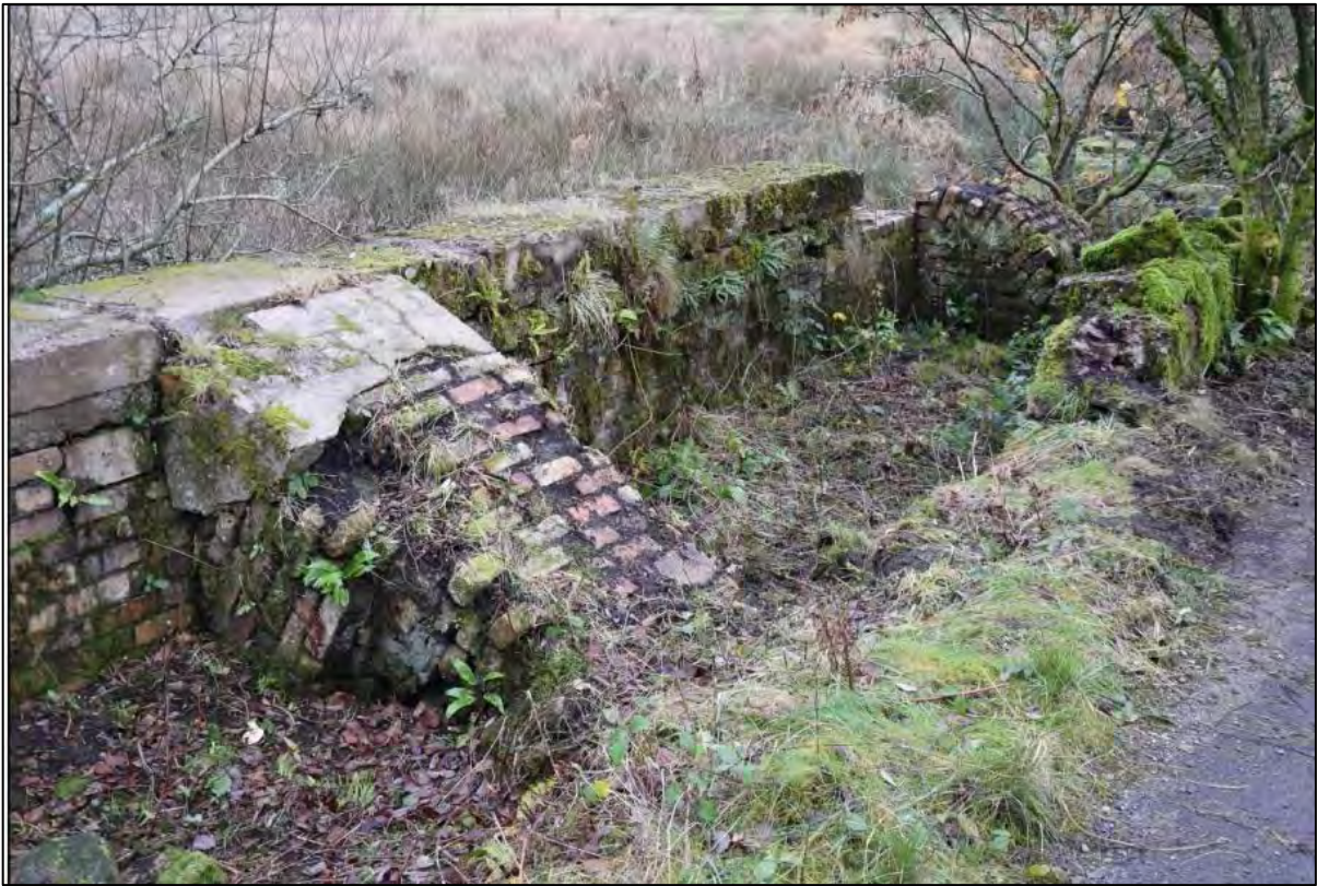
Figure 2.7: The remains of the brick and stone weir at Walkmill Community Woodland
