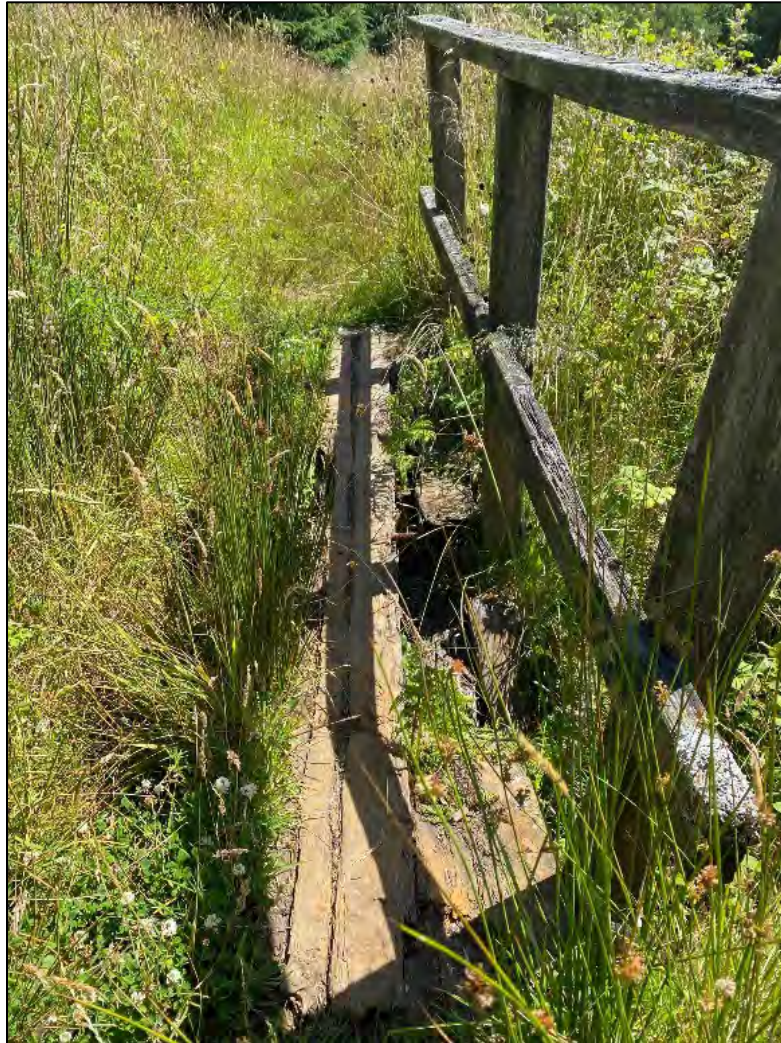
Figure 4.22: The broken bridge to the north east of the car park
