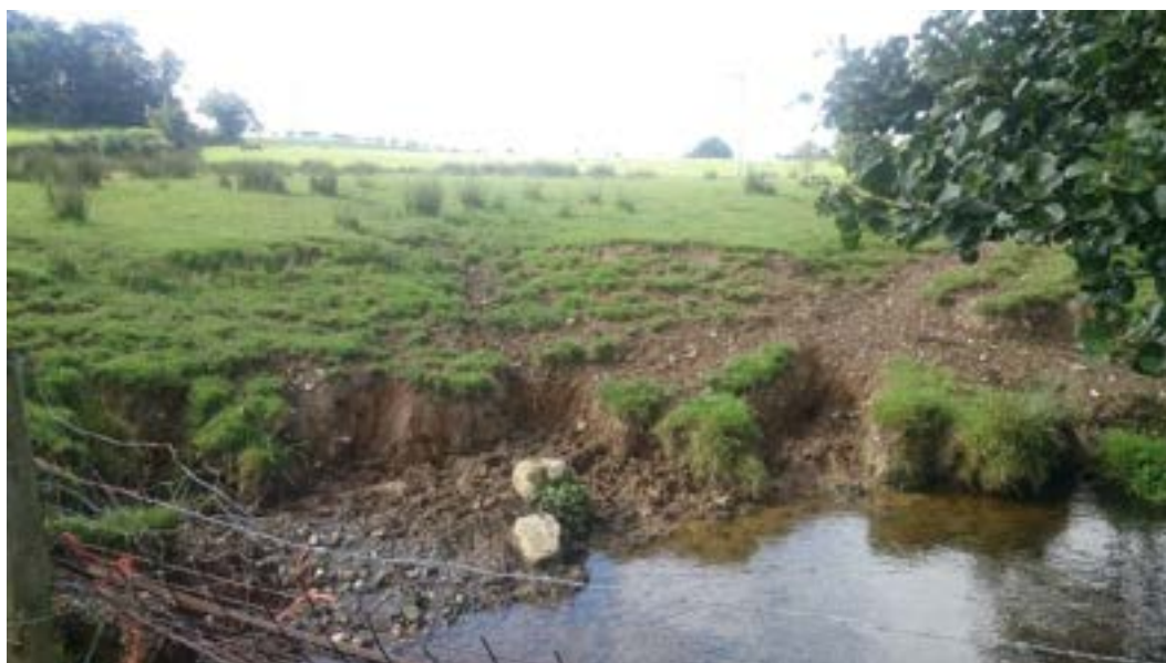
Figure 15. An example of a survey site classified as Repair, which currently has erosion problems caused by livestock access, but could easily be repaired with fencing and willow spiling or tree planting.
