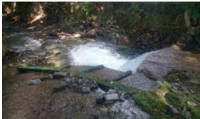
Figure 22: A photograph from 2016 of the drop between the concrete cap and the river bed on Liza Beck. Also shows the attempts at fish easement but this has since deteriorated further.
